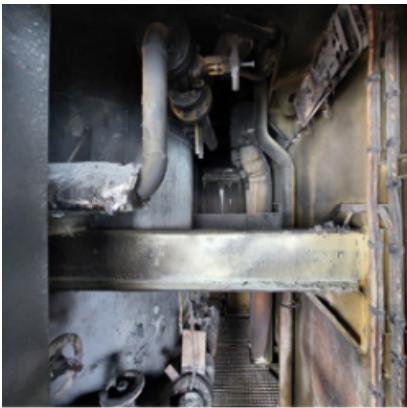
Figure 8: Starboard Engine Room Casing and Economizer post fire.
